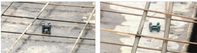
Fig. 4. Spacers which originated loose from the reinforcing, no longer accomplishment its purpose [13]
