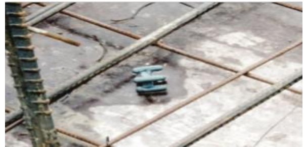
Fig. 5. Spacer that fell throughout a concreting process [13]
