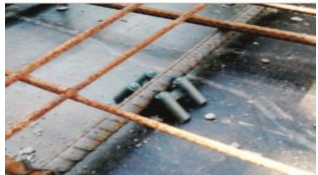
Fig. 6. Spacer deformation due to service loading [13]
